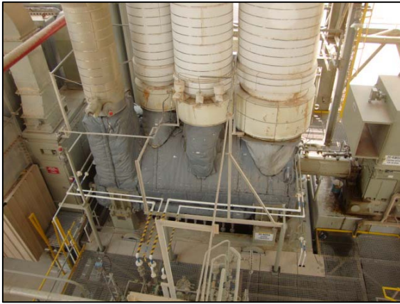
Figure 3: View of Propane Compressor at Train-2
