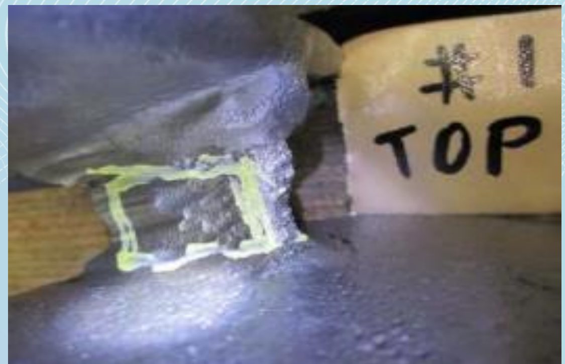
Eroded Vanes(top half)
