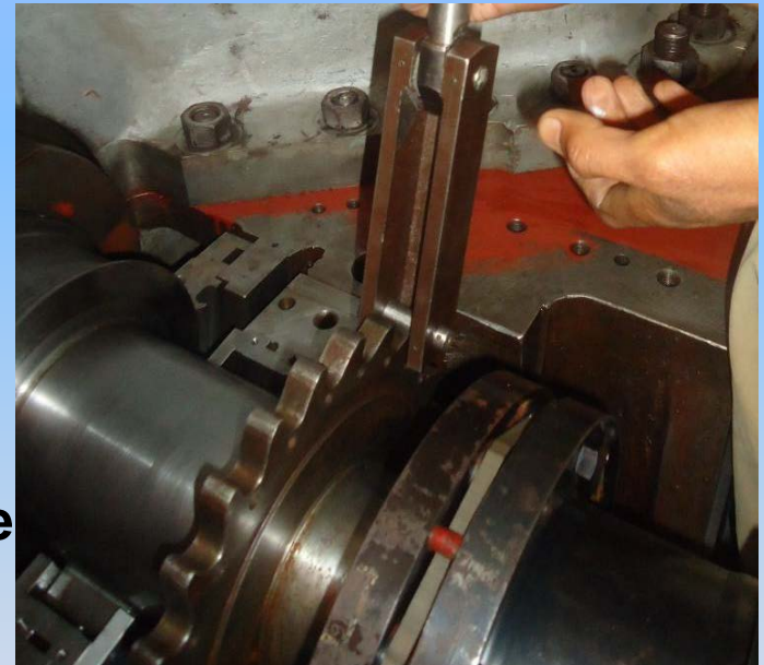
Exhibit # 3: Hydraulic barring latch arrangement (rotor could not rotate due to broken tooth)
