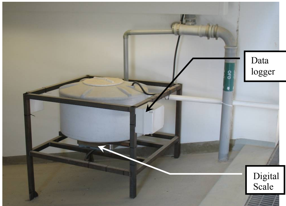
Figure 5. Condensate Collection System for AHU#6
