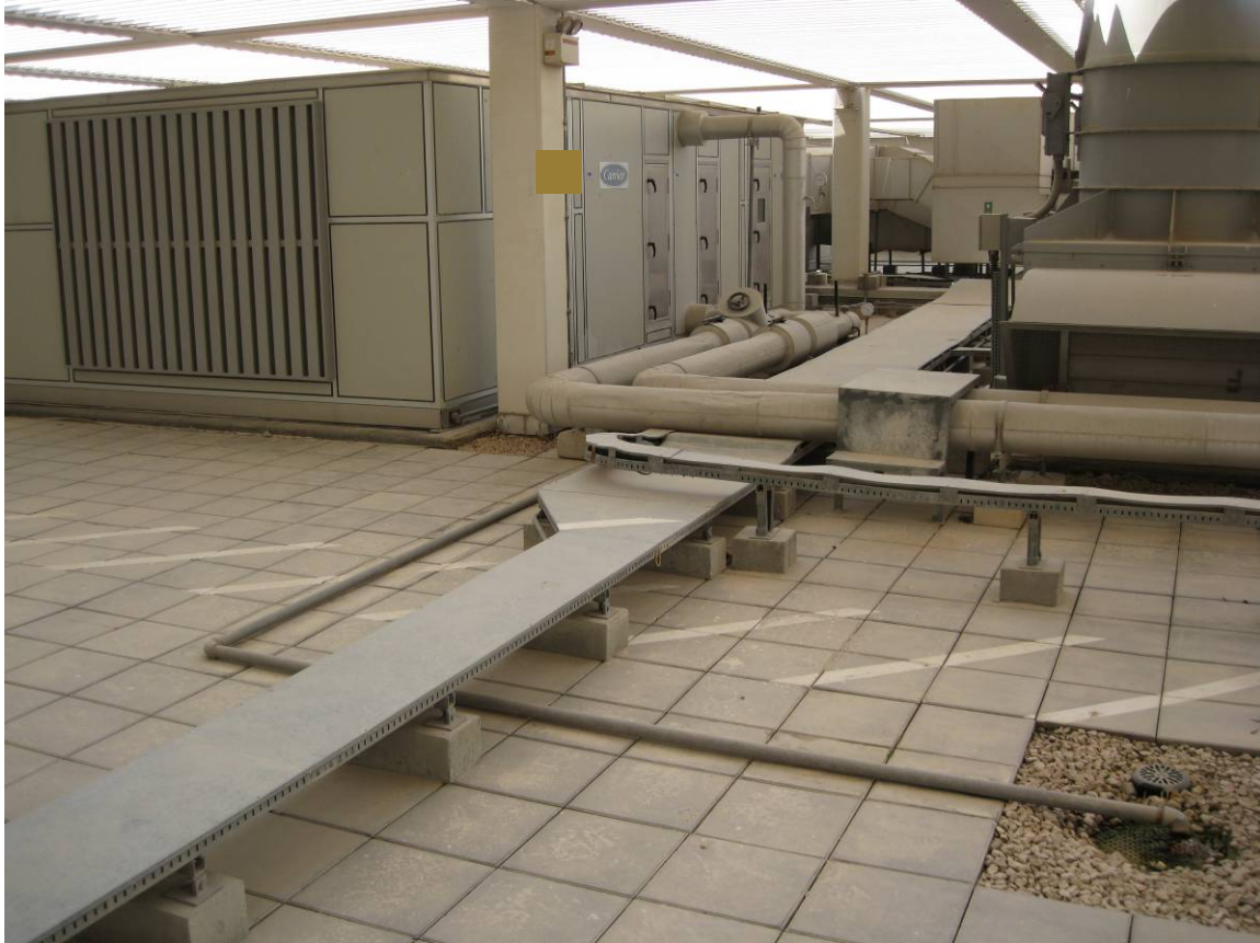
Figure 1. Condensate Piping from AHU to Roof Drain, Typical of all Units
