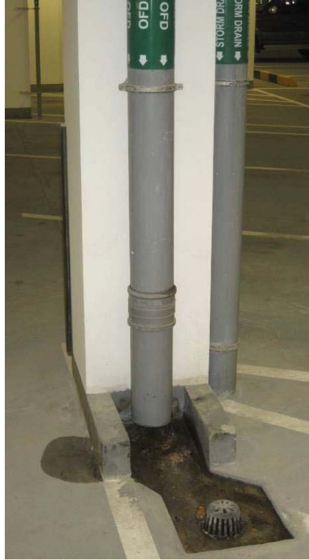
Figure 2. Floor Drain and Down Section of OFD Piping in Parking Garage, Typical for all Units.
