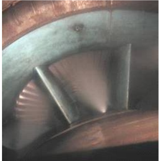
Figure #21 – Online Liquid Cleaning of Comp. Blading
