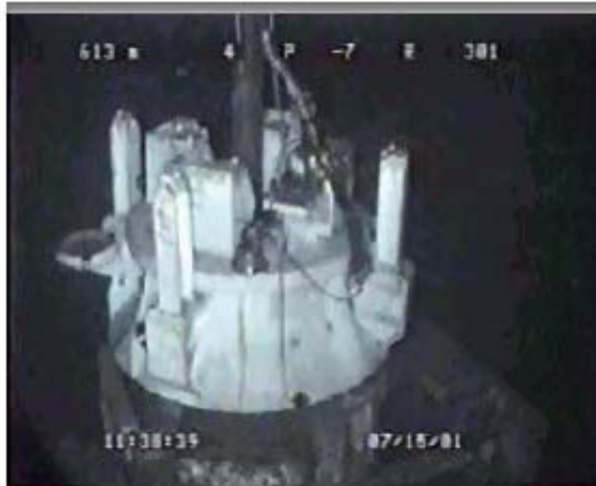
Fig. 2.5a- ROV photo of the TCRT on the Christmas tree prior to pumping the SGN fluids. 10
