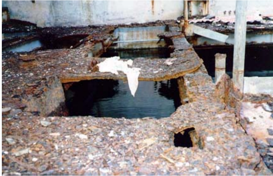
Figure 2.7 Uniform corrosion attack on structural steel [16].
