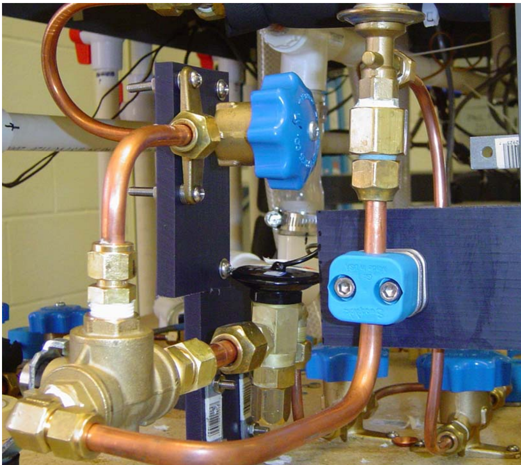
Fig. 2.17 Auxiliary expansion device manifold, evaporator #2
