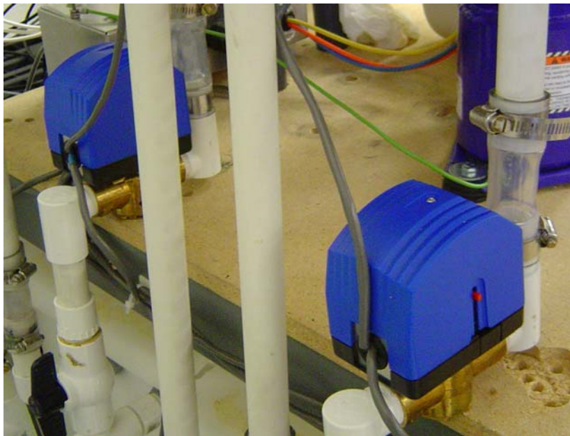
Fig. 2.23 Water flow valves
