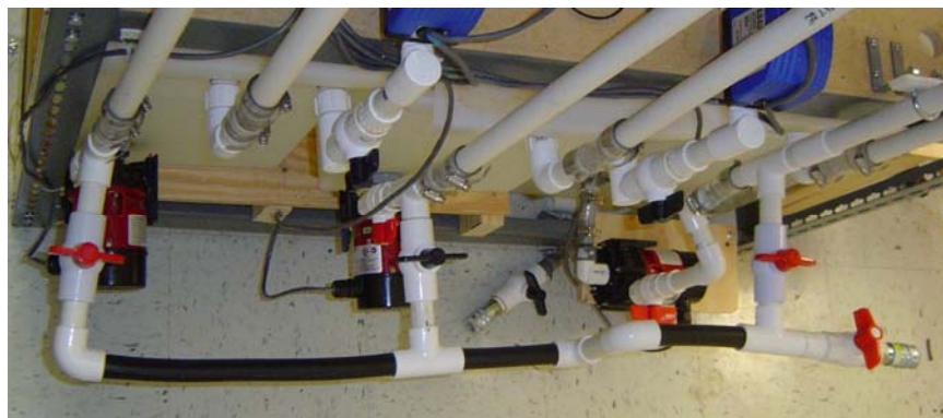
Fig. 2.8 Water pump manifold
