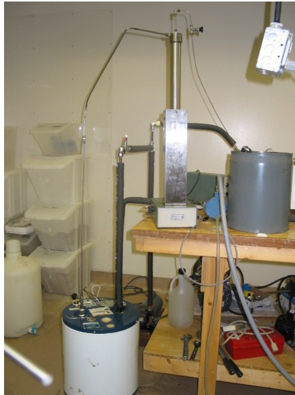
Fig. 4.20—Metering pump connected to the storage tank.
