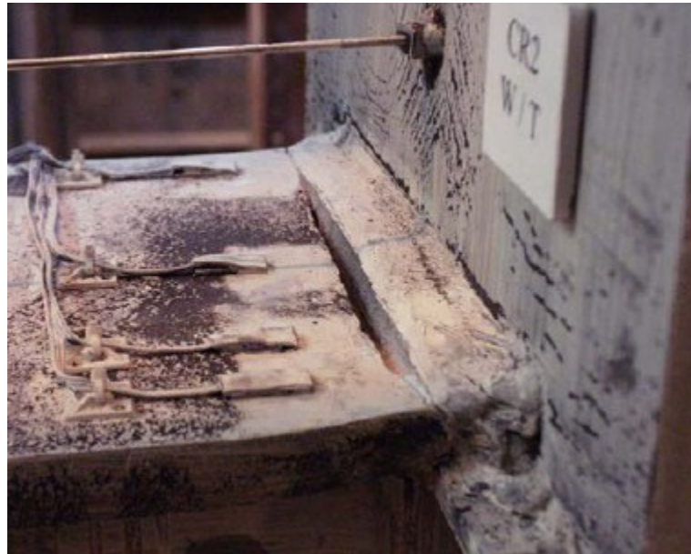
Figure 4.3 Beam flange fracture of CR2 (Lee et al. 2005(a))
