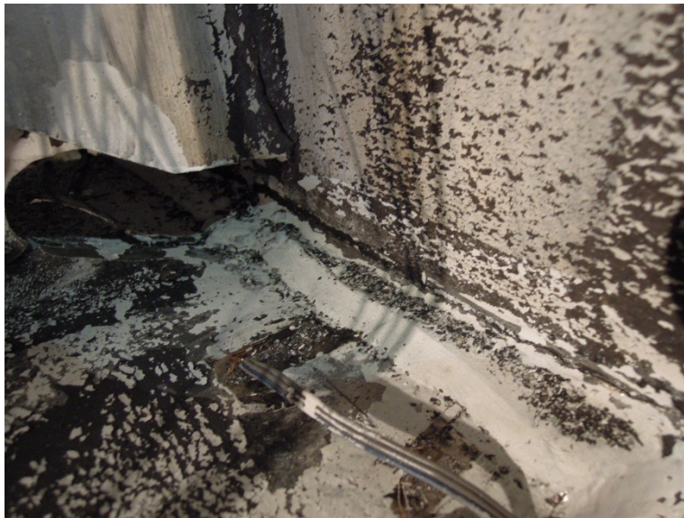
Figure 5.82 Photo of the west beam bottom flange of Specimen 4 after the second loading cycle of 6% drift ratio
