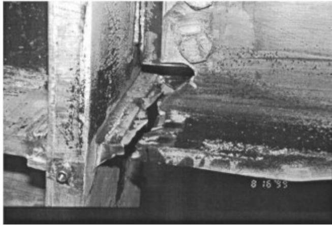
Figure 1.3 Fracture near beam flange groove welds of a weak panel zone (Engelhardt et al. 2000)
