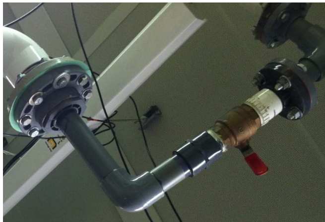
Figure 4.7. Separator Air Exit Ball Valve
