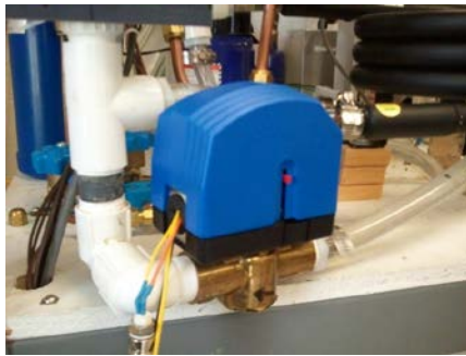
Figure 2.12: Water flow valve
