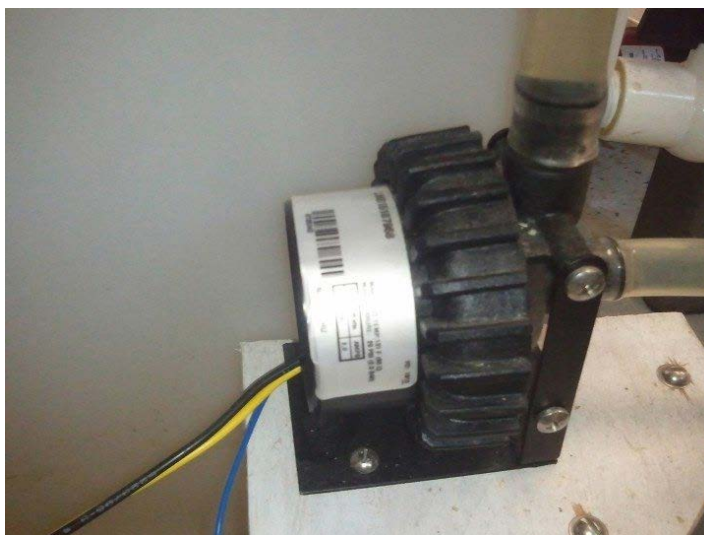
Figure 2.11: Condenser water pump
