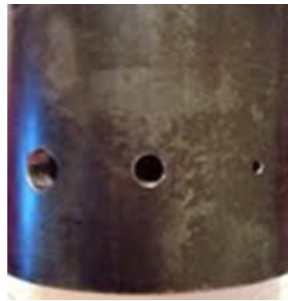
Figure 8: Holes Drilled on the Same Cross-Section of a Pipe
