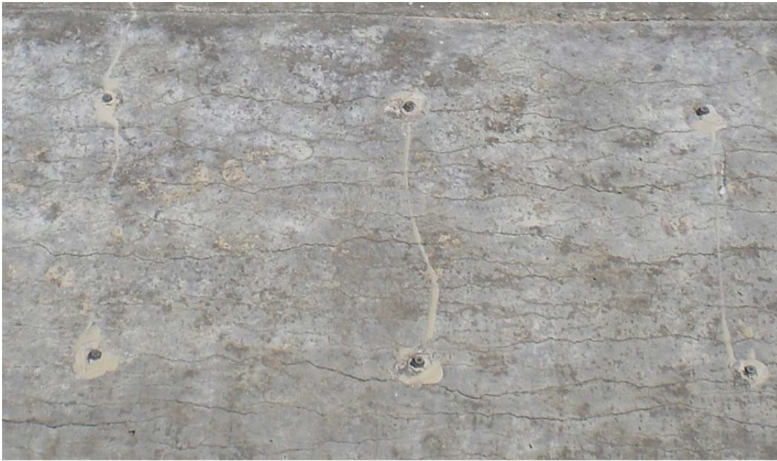
Figure 3-15. Longitudinal Cracks from ASR Expansion.
