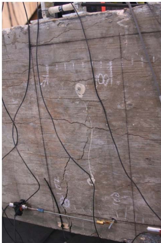
Figure 5-30. Flexural Crack under Actuator 1 during Four-Point Test for LSC5.
