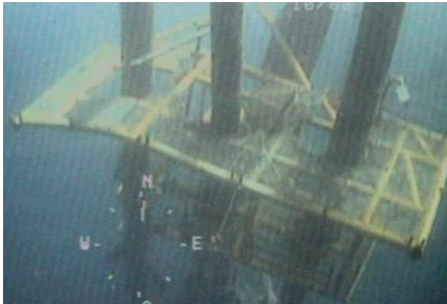
Fig. 1.1—Platform was destroyed by hurricane Ike in the East Cameron Area. (BOEMRE, 2010)
