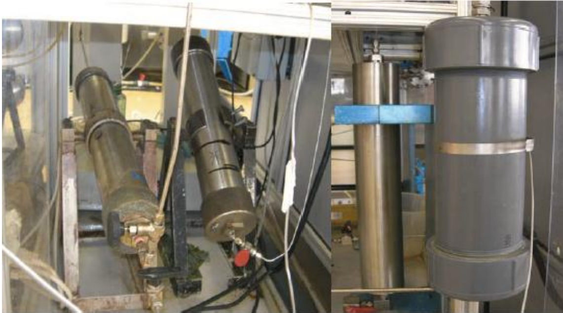
Fig. 2.9—Water Accumulator and Refilling Tank
