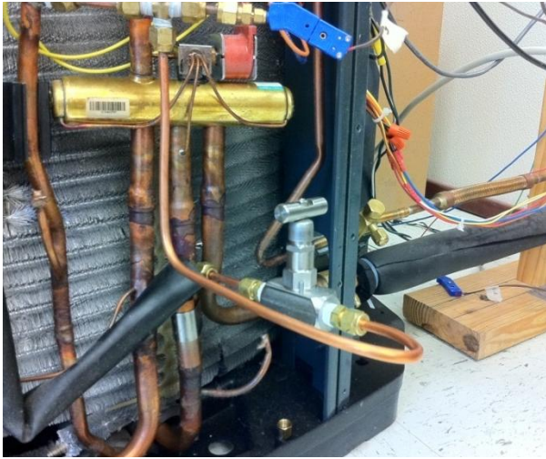
Figure 4.14 Bypass Valve Installed on the TRANE System
