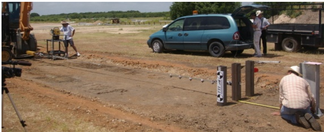
Figure 3.127. Static load test on group of posts system embedded in hard clay
