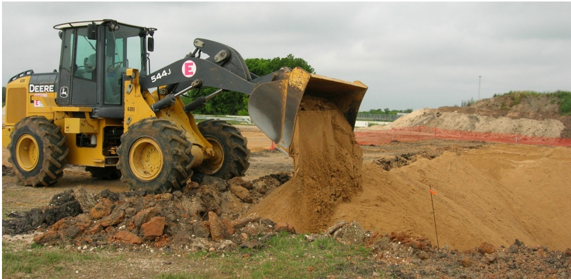
Figure D.2. Dumping clean sand into the excavated ditch for the impact test
