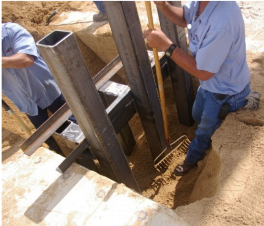
Figure 3.73. Installation of a group of posts system with two by three group of posts
