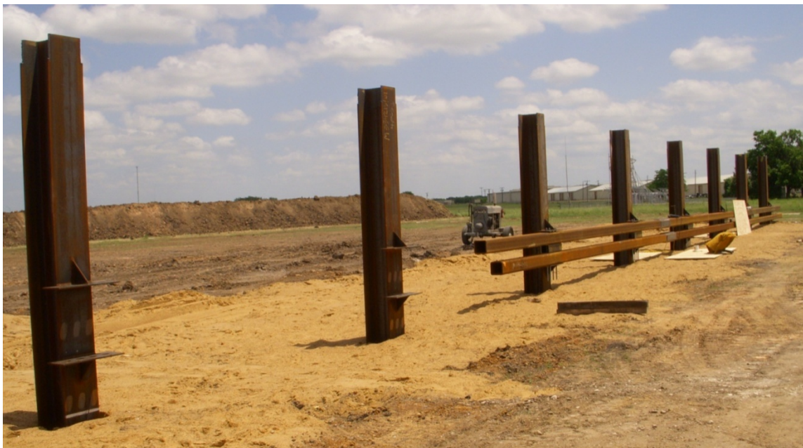
Figure D.3. Installation of horizontal beams of the group of posts system
