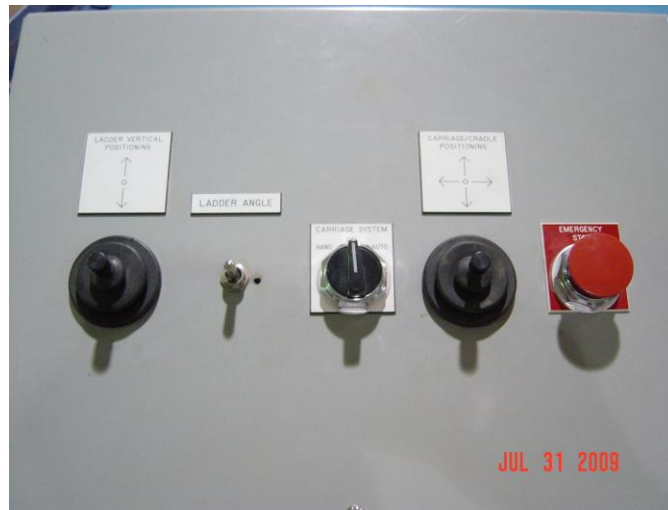
Figure 5. Picture of Manual Dredge Controls
