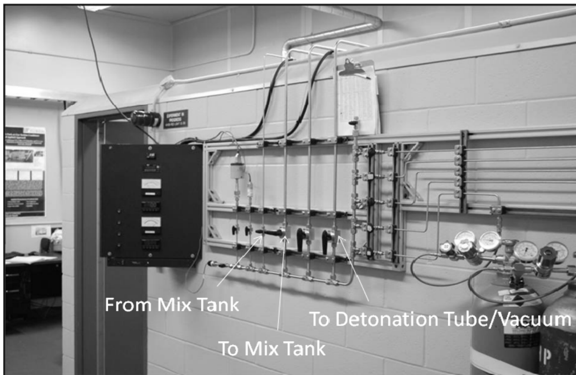
Figure 26 Photo of the mixing manifold outside of the blast wall.
