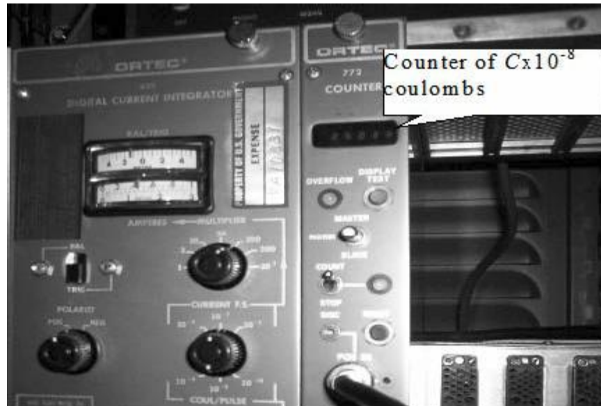
Fig. 2.10 —Counter panel located in the control panel reads charge of electrons passing through the parallel plate transmission ion chamber.
