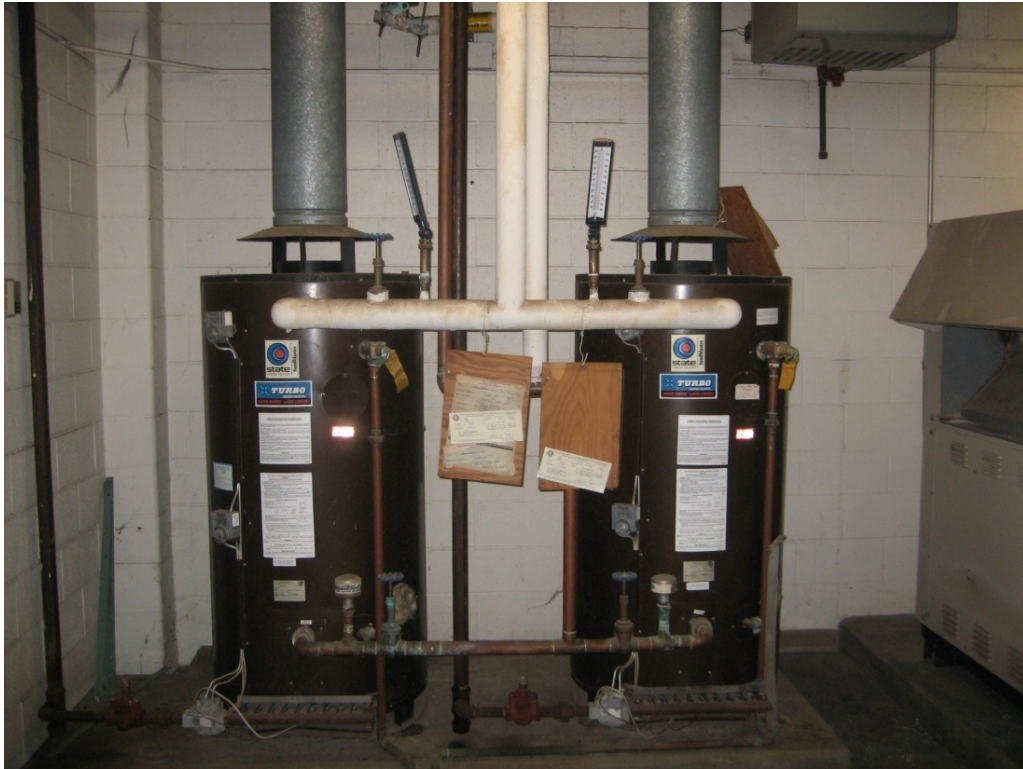
Figure 5.3 - Service Water Heaters for the Case-study School
