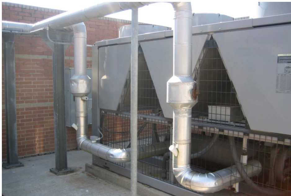
Figure 5.1 - Air-Cooled Scroll Chiller for the Case-study School
