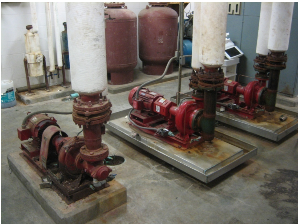
Figure 5.4 - 2 Pumps for Chillers (2) and for Boiler (1)
