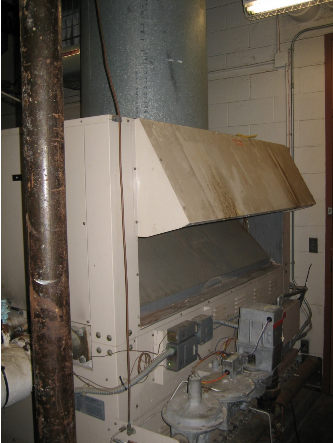
Figure 5.2 - Hot Water Boiler for the Case-study School
