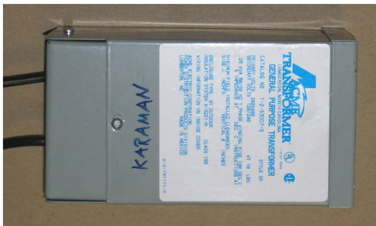
Figure II.7. ACME step-up transformer used to increase the voltage supplied to heaters.
