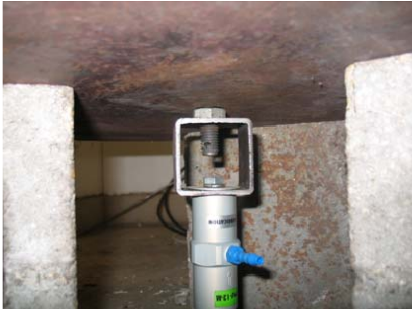
Figure A-5 pneumatic vibrator of variable frequency coupled to the grate and placed under the plenum
