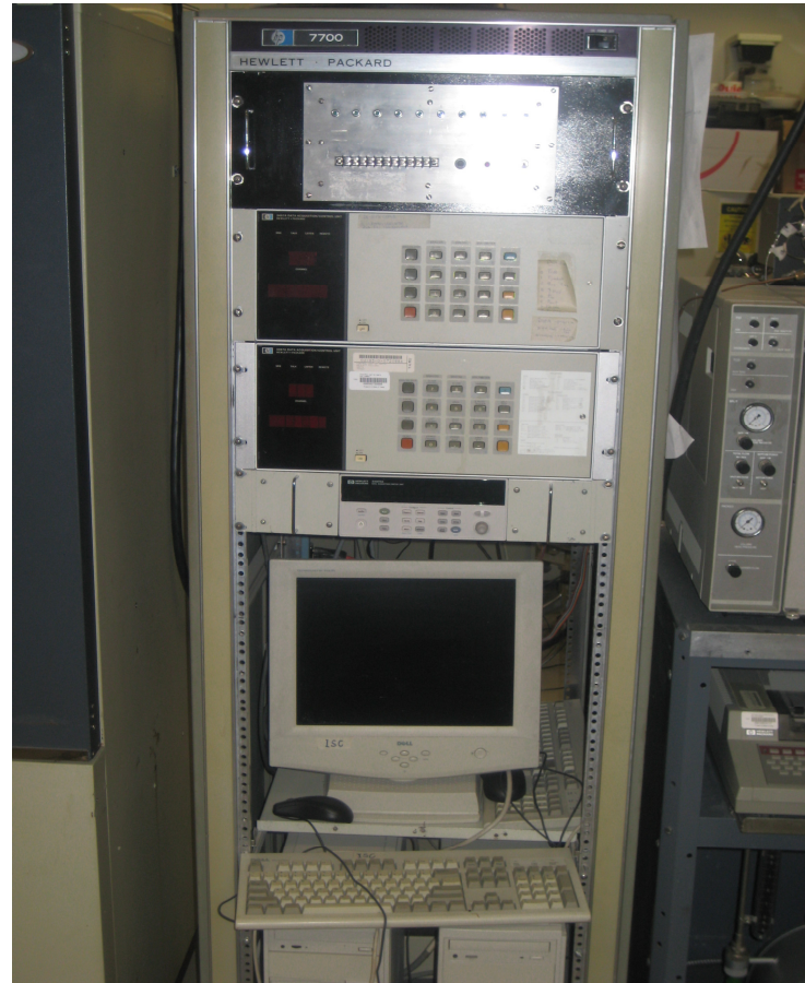
Fig. 3.11—Data logger unit and PC.
