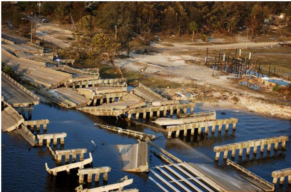
Fig. 1 Highway 90 bridge damaged during Hurricane Katrina. The bridge was located on US-90 in Biloxi and Gulfport, Mississippi Gulf Coast (From Gulf Coast Information System (GCIS, 2006)
