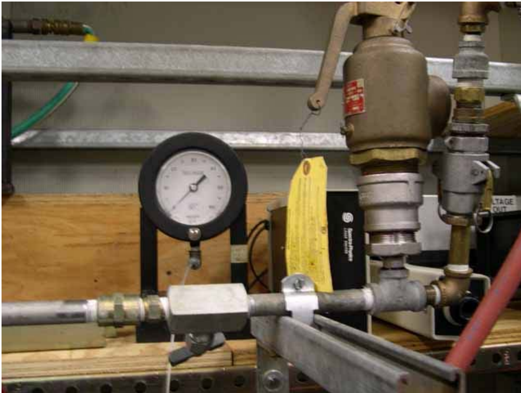
Figure A8. Air Flow Rate Control Valve, Inlet Pressure Gage, and Safety Release Valve
