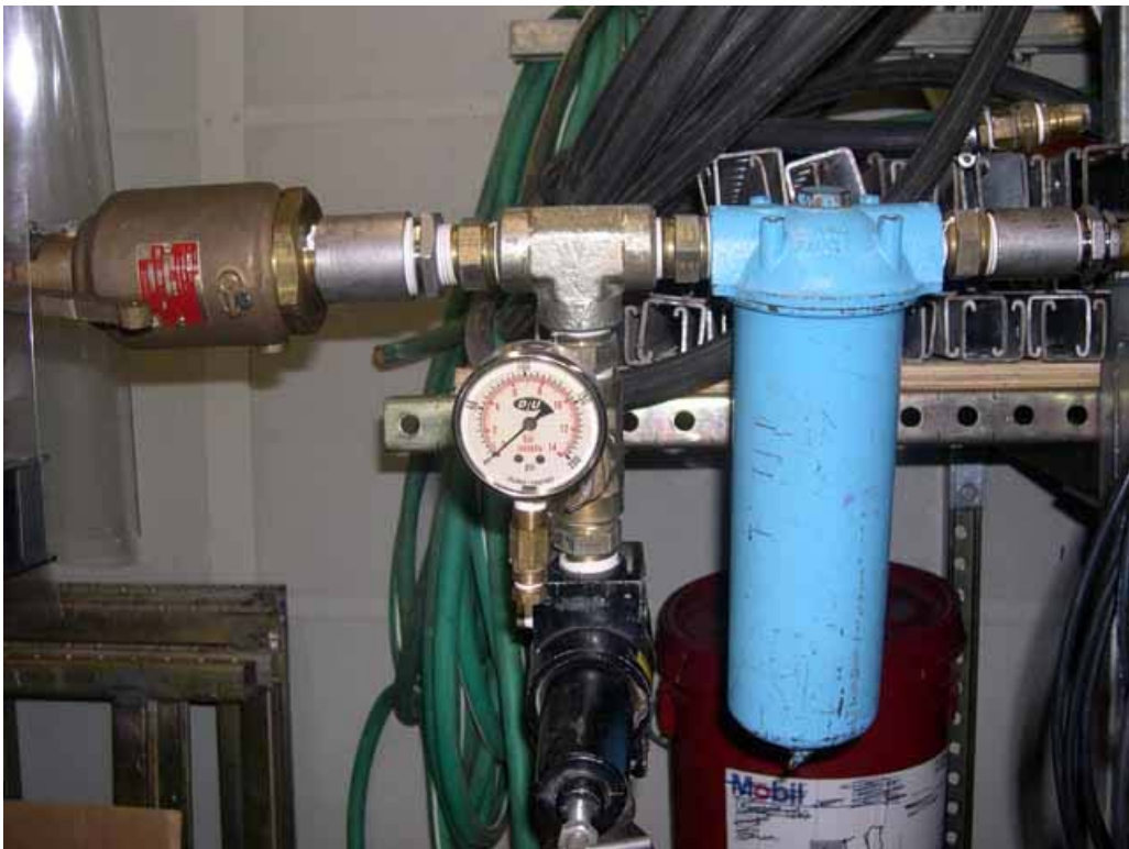
Figure A5. Regulator, Safety Release Valve, and Air Filter
