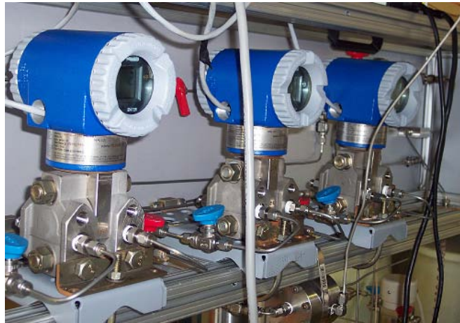
Figure 3.22 Pressure transducers and there connections
