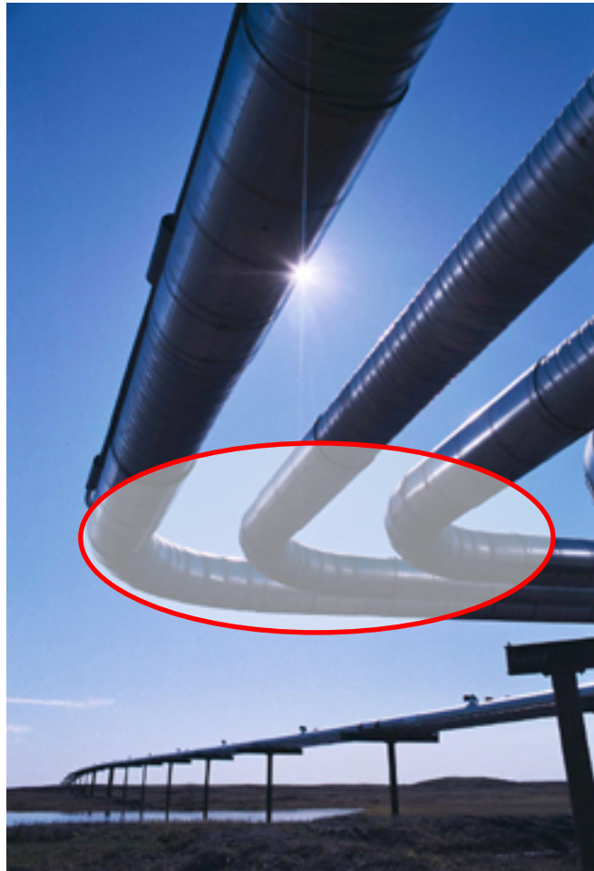
Fig 3.9 - Pipe bends which are potential areas for erosion
