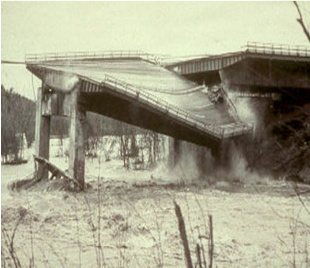
Figure 7-5. One of the Schoharie Creek Bridge spans plunging into the river.
