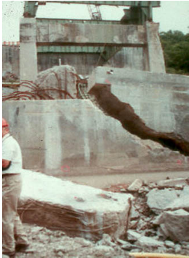
Figure 7-11. Photo of Pier 3 taken in 1987 after the failure.
