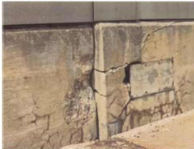
Figure 2.3 Misalignment of Adjacent Sections of a Parapet Wall on a Highway Bridge Due to ASR (Strategic Highway Research Program (SHRP)-315, 1991).
