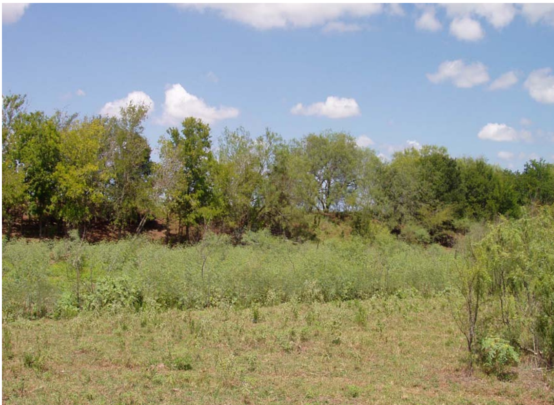
Figure 6.5. River Side of Repaired Burleson County Levee. The earthen levee was constructed of soil dug from a borrow pit immediately adjacent to the levee and on its river side. At this location in mile 10 of the levee, the borrow pit is overgrown with vegetation that is distinct from the scrub brush and mesquite in the foreground. The borrow pit was originally 3 to 4 feet deep, 318 but is now 1 to 2 feet deep. The levee can be seen along the horizon, immediately behind the treeline that has grown up on its river side. Photo by the author.
