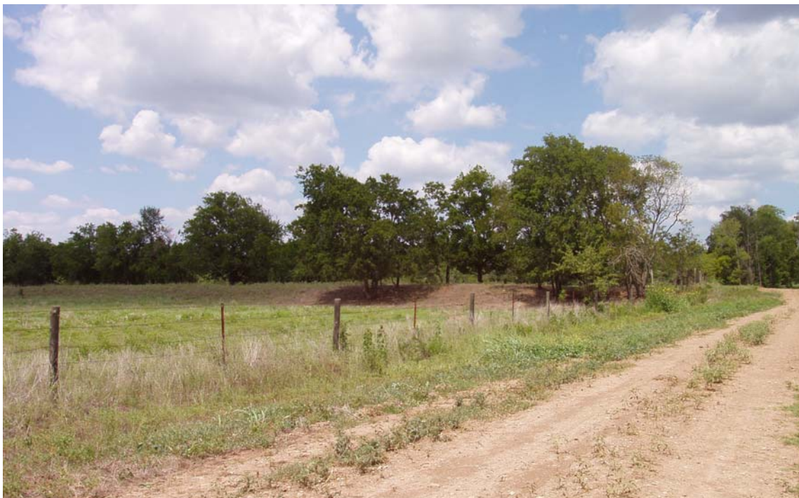
Figure 6. 4. Land Side of Original Burleson County Levee. View to the northeast on County Road 277, formerly Batte’s Ferry Road. The levee is from mile 20 of the improvement project in a location that is largely intact from its original construction. The levee is 3 to 4 feet high. There is more vegetation on the river side of the levee than on the land side of the levee because water collects in the slightly lower borrow pit on its river side. The river is 750 feet beyond the levee. The original plan specified the levee would be constructed “on the west bank of river at a distance of 200 to 1000 feet in order to cut off bends and avoid caving banks.” 317 Photo by the author.
