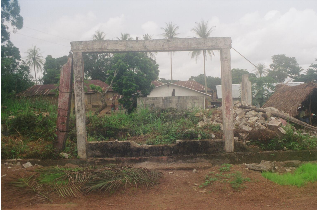
Figure 31: Remains of a Destroyed House in Blama
