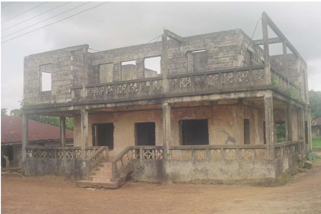
Figure 32: Remains of a Looted Office in Blama
