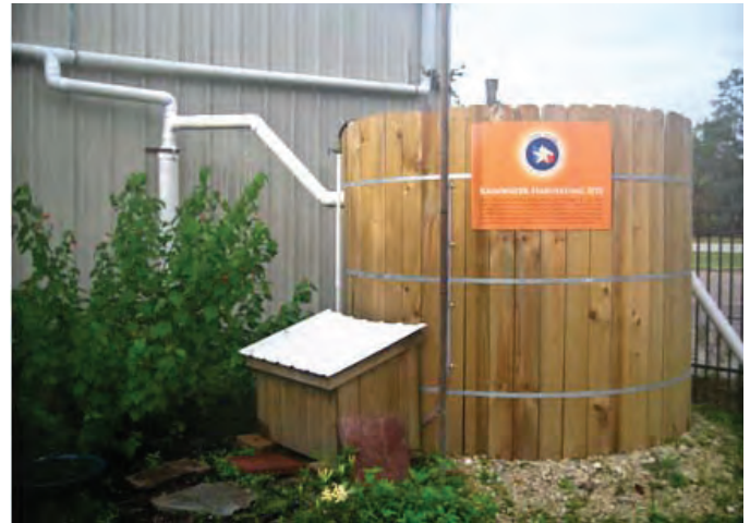
Rainwater harvesting system
