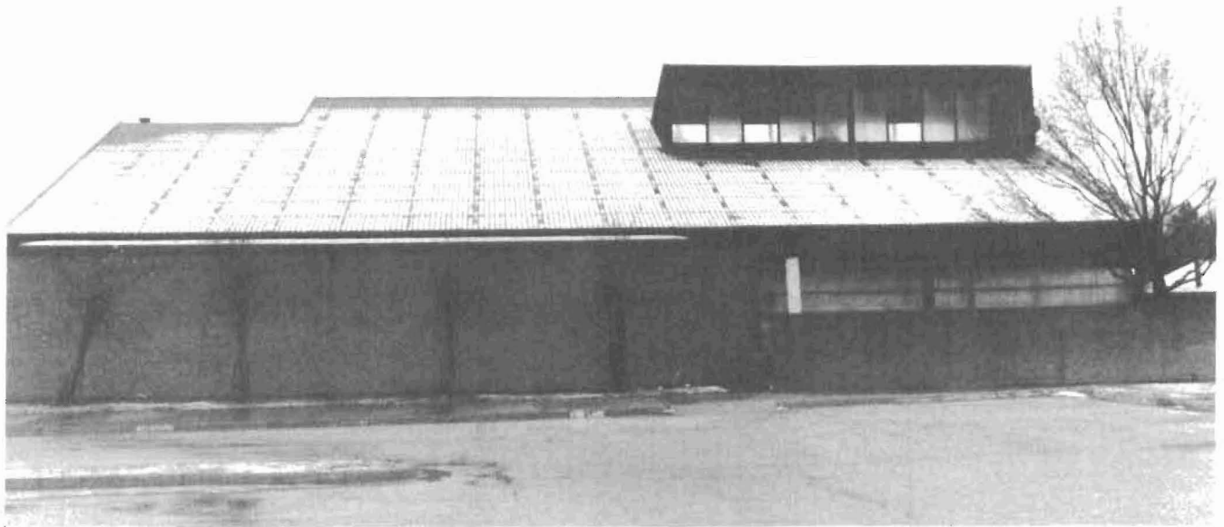
Figure 2. Melting snow indicates major points of winter heat loss and initial locations of concealed condensation in metal roof assembly with stapled insulation seams.
