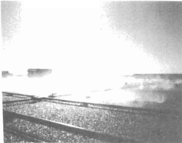
Figure 3 Roof Cooling System in Operation (Photo courtesy of Fan-jet Cooling Systems, R. R. Abernethy, Inc., Carrollton, TX)
