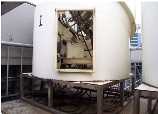
Fig. 3 Corrosion of the body
