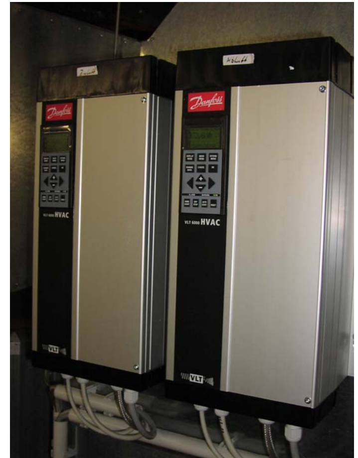
Inverters for supply and exhaust air ventilators
