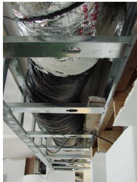
Figure 6 MHLab soffit duct (supply side).
