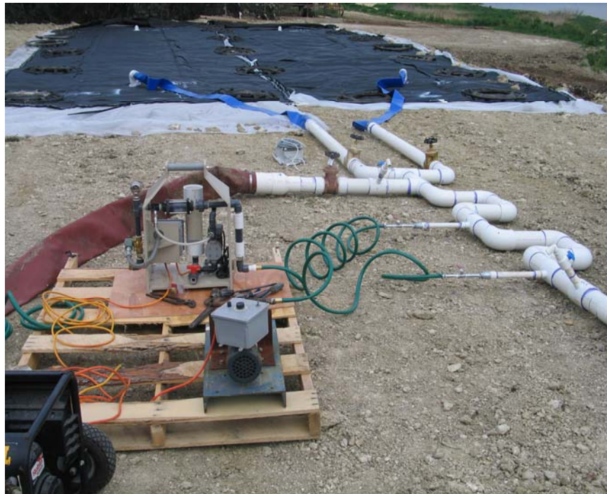
Figure 1. Geotube ® dewatering system prior to treatment
