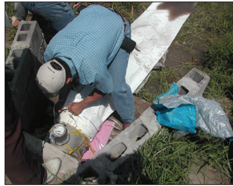
Figure 4a. Poly-pipe connected tightly to the supplying pipe.
