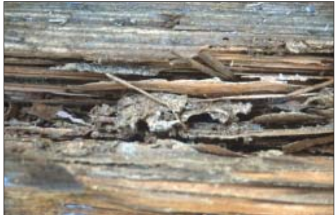
Figure 10. Termite damage in wood.
