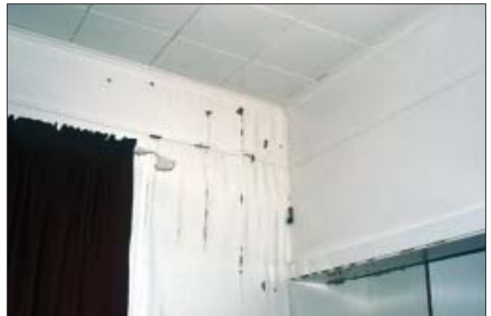
Figure 12. Shelter tubes on interior walls.
