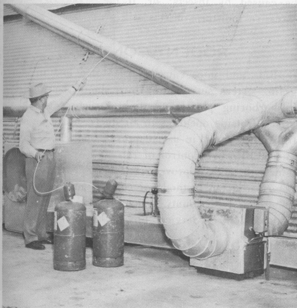
Figure 12. Large buildings generally can be fumigated more economically with gas-type fumigants. Here the fumigant is introduced into a duct and recirculated by means of a small fan.
