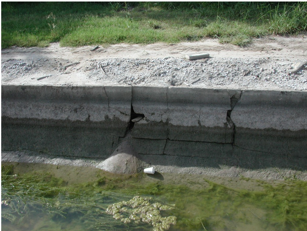
Figure 1. Large cracks and aquatic vegetation shown above contribute to higher total losses of canal segments.
