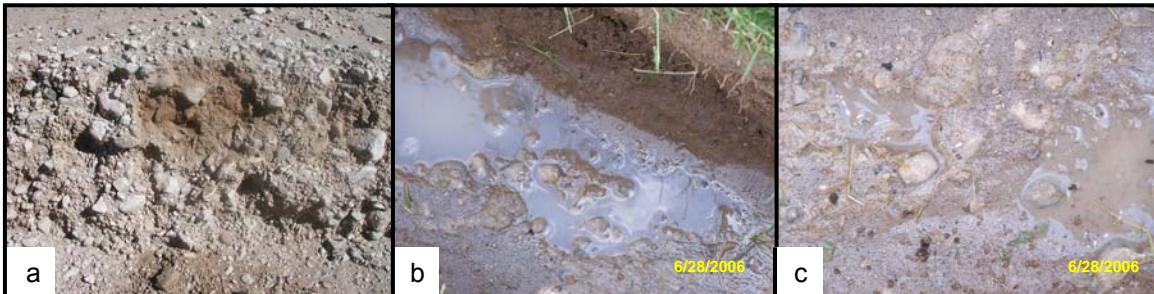
Fig. 6 A typical Canutillo gravelly loam and water ponding over the subgrade.
