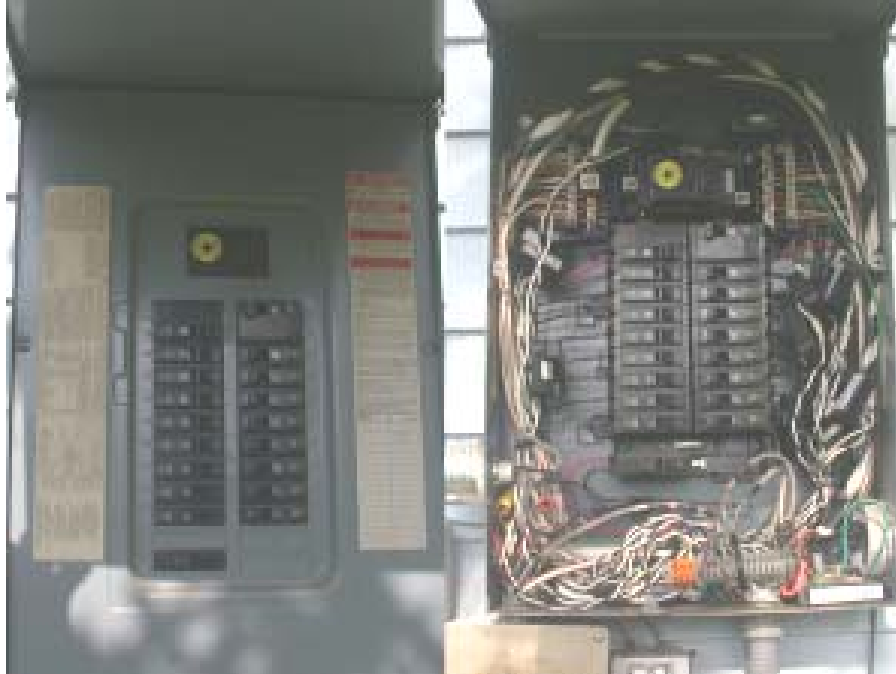
Figure 177: Electrical panel with the current transducers, face on (left) and face off (right) (Source: Kim 2006)
