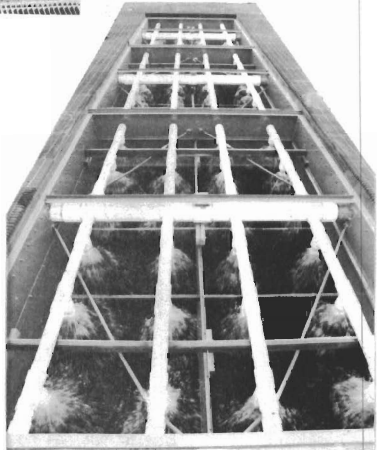
Figure 5 - By changing 388 small orifice nozzles to 36 non-clogging square spray type and installing cellular fill, 5°F colder water was obtained.
