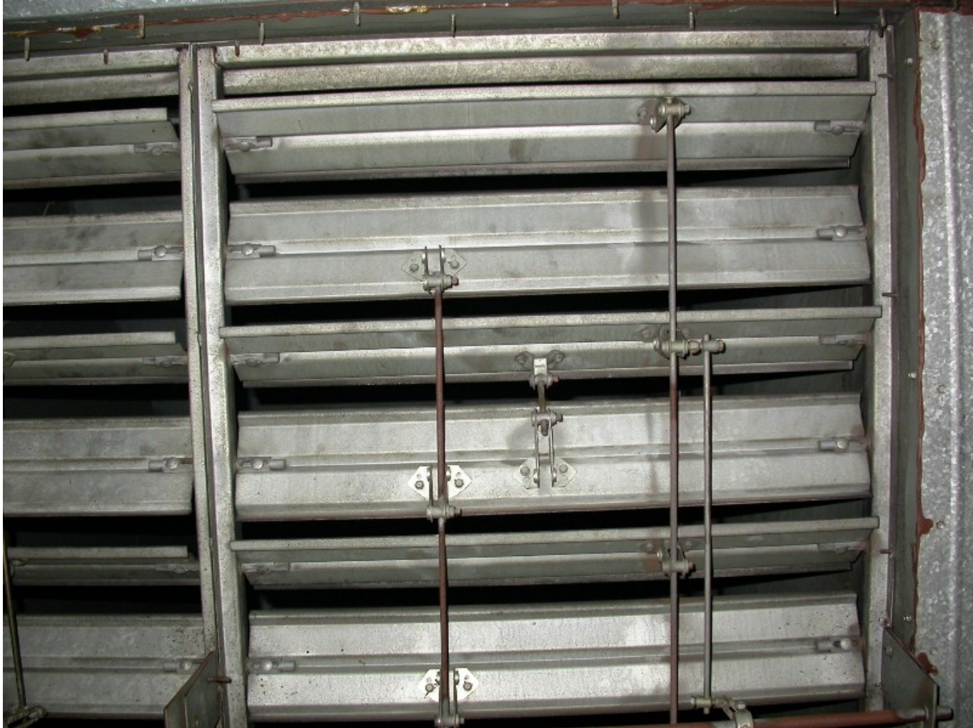
Bypass Damper Original condition, fully open
