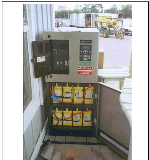
Figure 5 – Inverter system with battery backup
