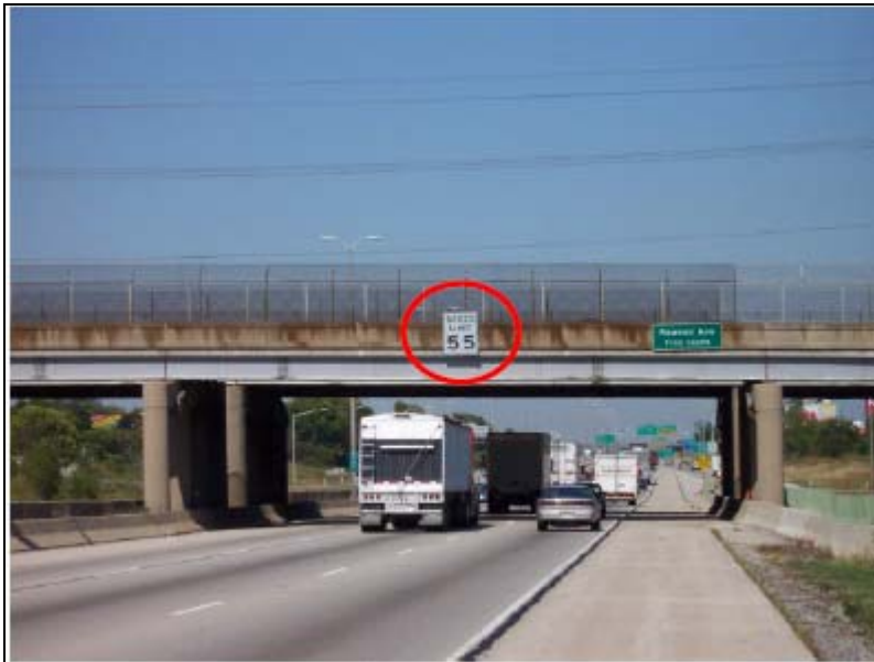
FIGURE 2 Overhead Speed Limit Sign (5).
